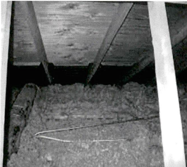
Preformed baffles installed in every joist cavity full width of the cavity.
