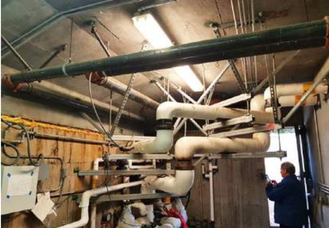
Articulated mechanical services : white pipes – arrangement with 3 ball joints
