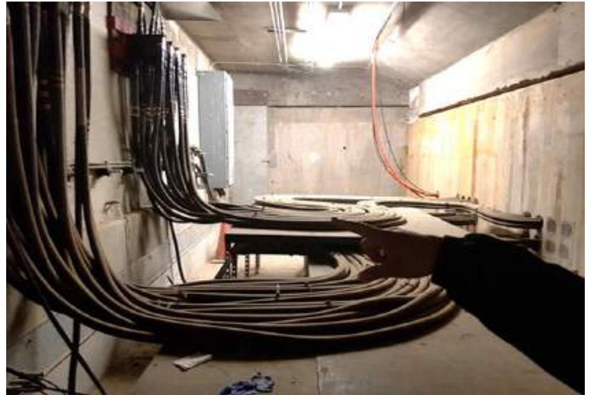
Electrical cables with movement allowance – slack on tables
