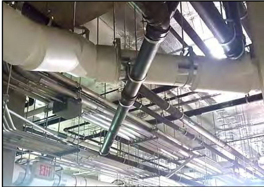
Ducts and other building systems
