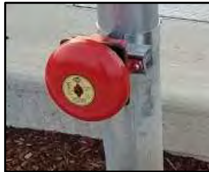
Exterior Alarm Bell
