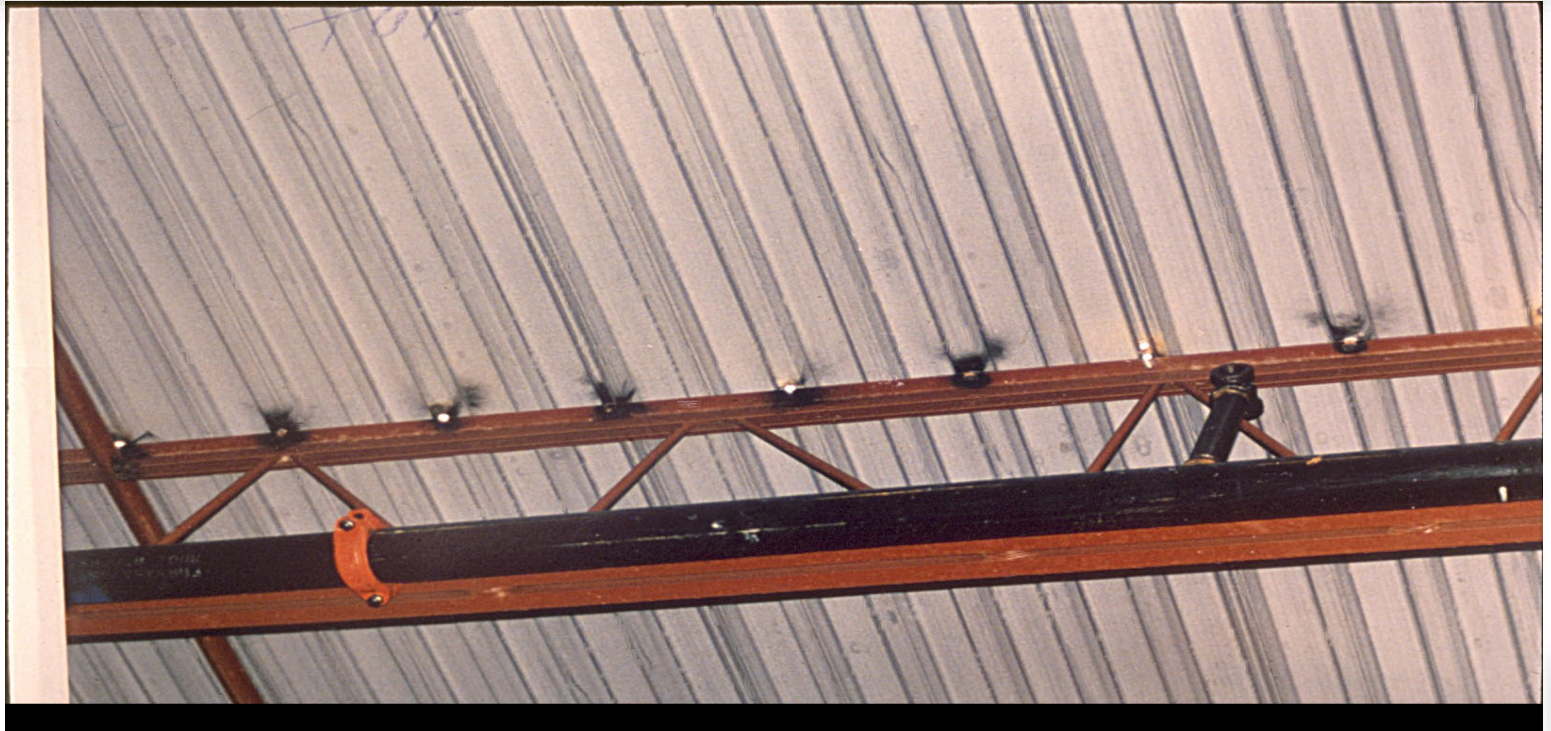
Damaged joist / deck
