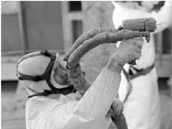
SPF products are commonly used in residential, light commercial, commercial, institutional, and certain industrial applications. Closed cell SPF (ccSPF) is applied to the interior or exterior side of the building envelope.
