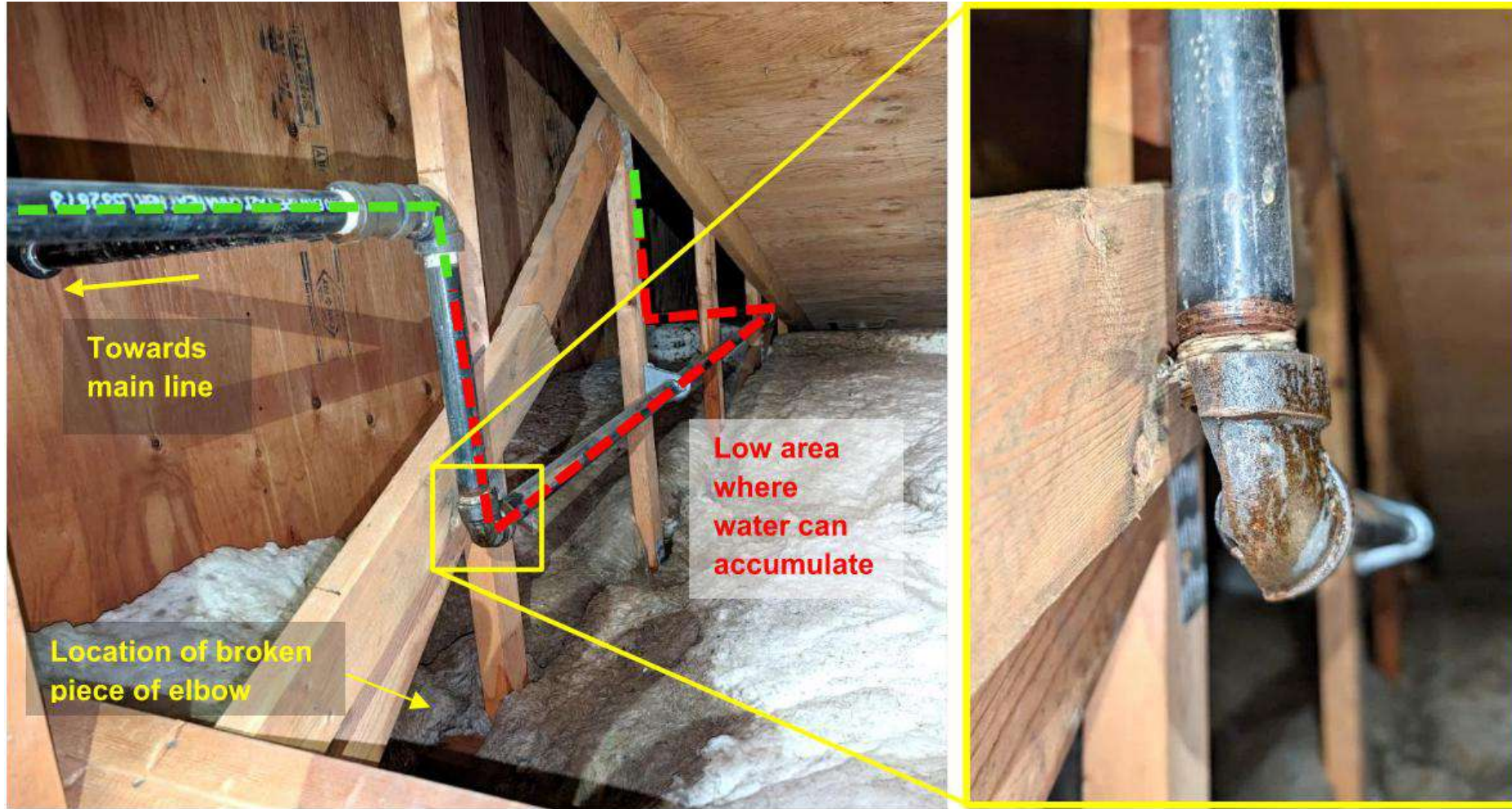
Figure 11: Photo of original installation annotated to show low points and broken piece of pipe elbow.
