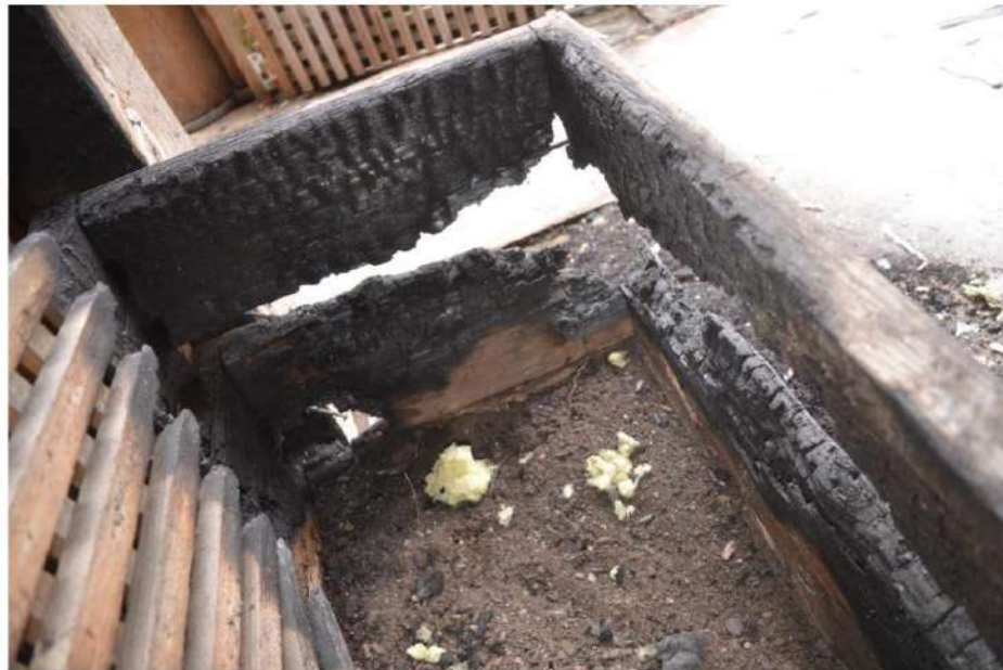
Figure 4: Concentrated charring to the inside of the planter box.
