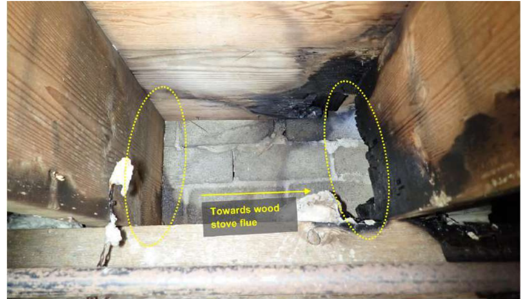
Figure 8: Charring to wood against corner of column with wood stove flue. Framing is immediately against the column.
