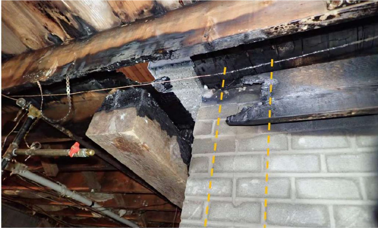
Figure 5: Dominant fire damage surrounding corner of column with wood stove flue.
